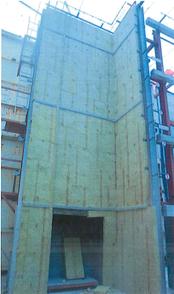
DLP C2858/1112 Cavity barriers and insulation
